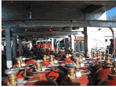
Figure 2 Pigtails used for an installation of bundles of cylinders
